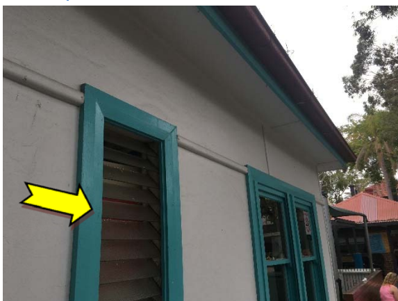
Photo 11. Exterior, throughout, window frames – suspected lead-containing blue upper paint systems.
