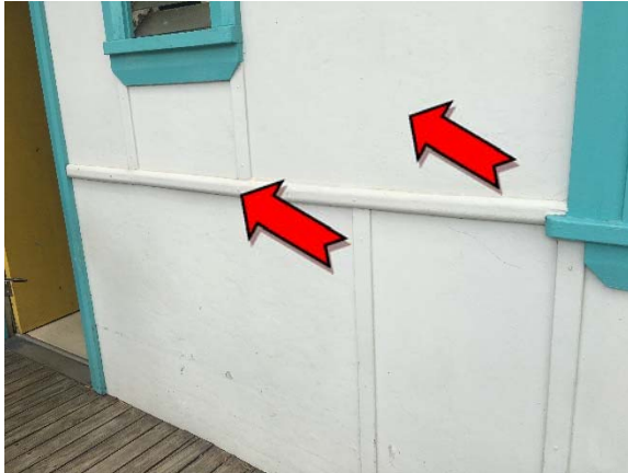
Photo 1. Exterior, throughout wall beading and walls – asbestos-containing moulded fibre cement and fibre cement sheeting and suspected lead-containing white upper paint systems.
