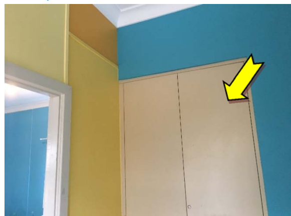
Photo 12. Interior, throughout, walls – suspected lead-containing blue and yellow upper coloured paint systems.
